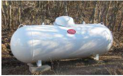
New Propane System
